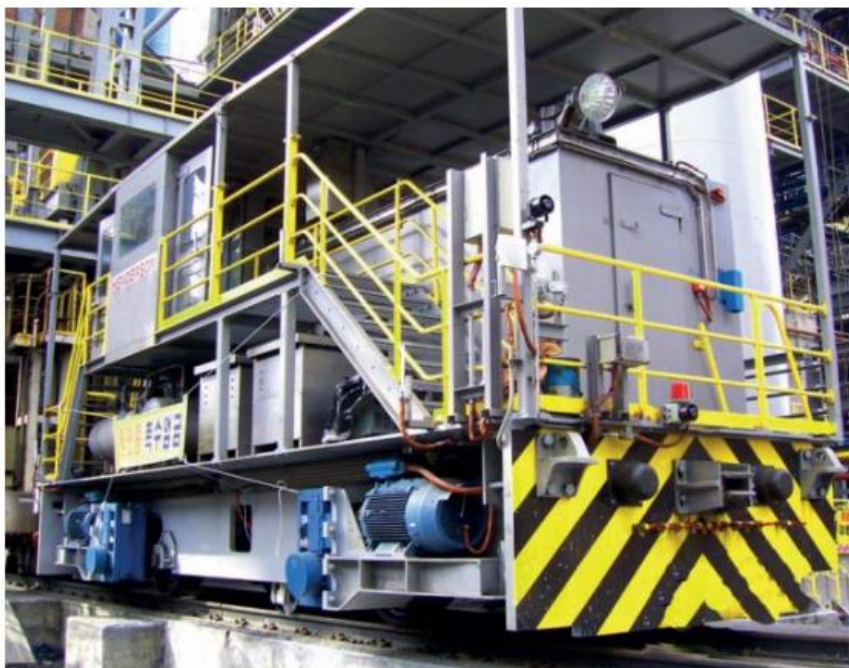
JMH Anti-Collision System installed on a Coke Locomotive
